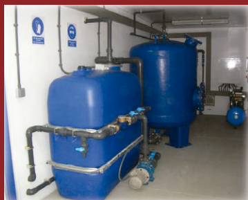
Filtration equipment 50 m 3 /h
